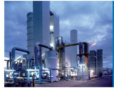
Air Liquide air separation unit
